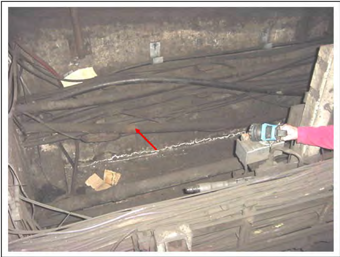
Figure 28: Material Strongly Presumed To Contain Asbestos
