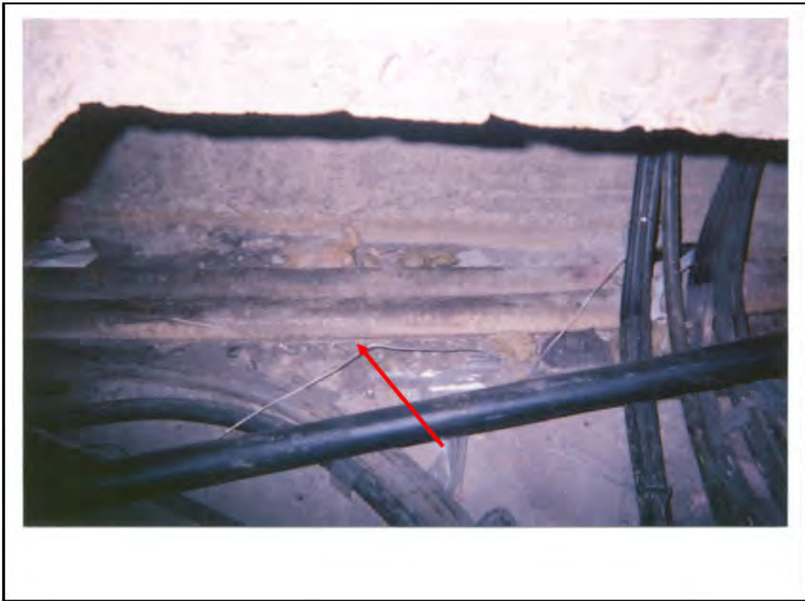
Figure 13: Material Strongly Presumed To Contain Asbestos
