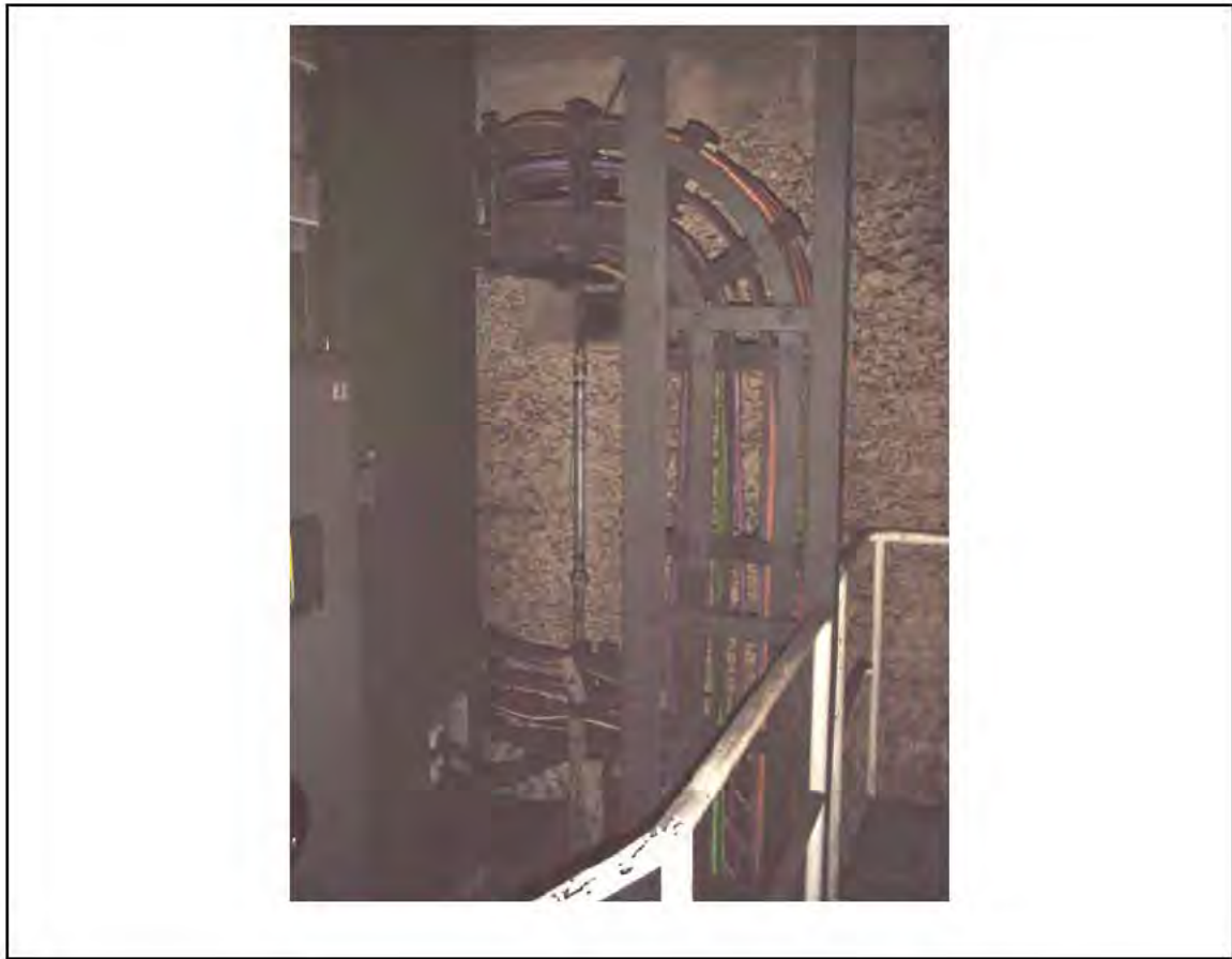
Figure 21: Material Strongly Presumed To Contain Asbestos
