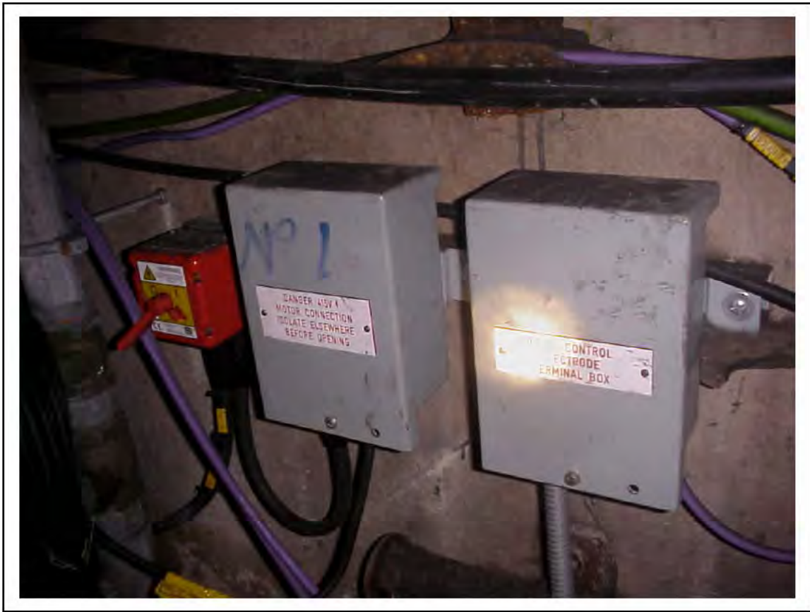
Figure 32: Material Strongly Presumed To Contain Asbestos
