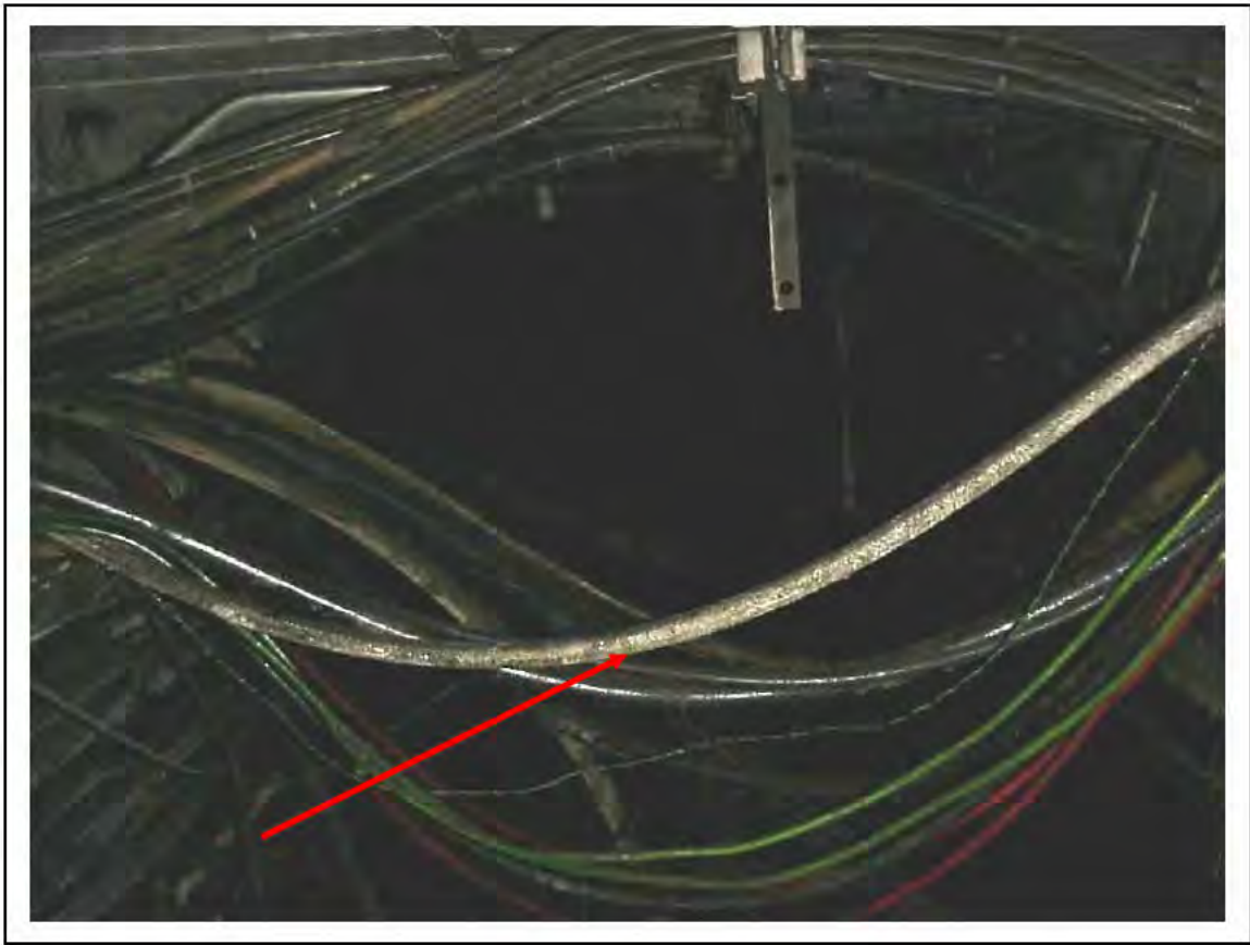
Figure 41: Material Strongly Presumed To Contain Asbestos
