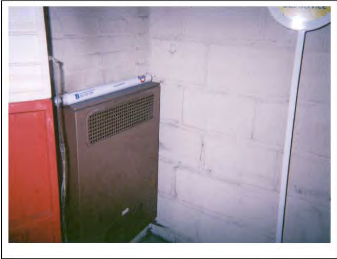
Figure 15: Material Strongly Presumed To Contain Asbestos
