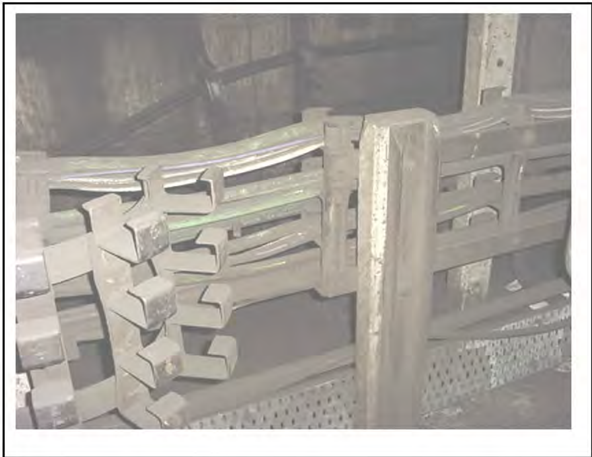
Figure 26: Material Strongly Presumed To Contain Asbestos
