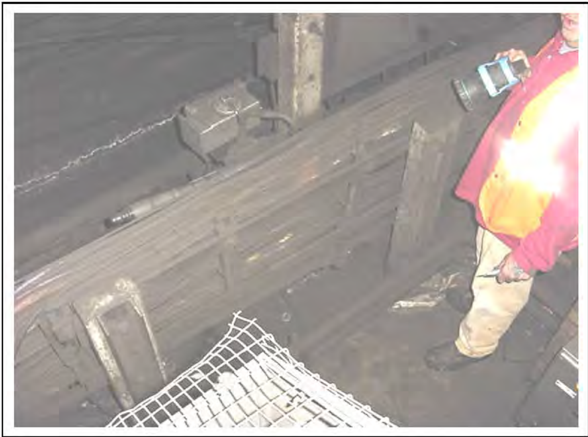
Figure 27: Material Strongly Presumed To Contain Asbestos
