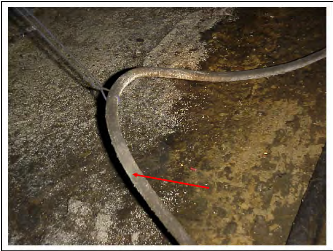
Figure 43: Material Strongly Presumed To Contain Asbestos
