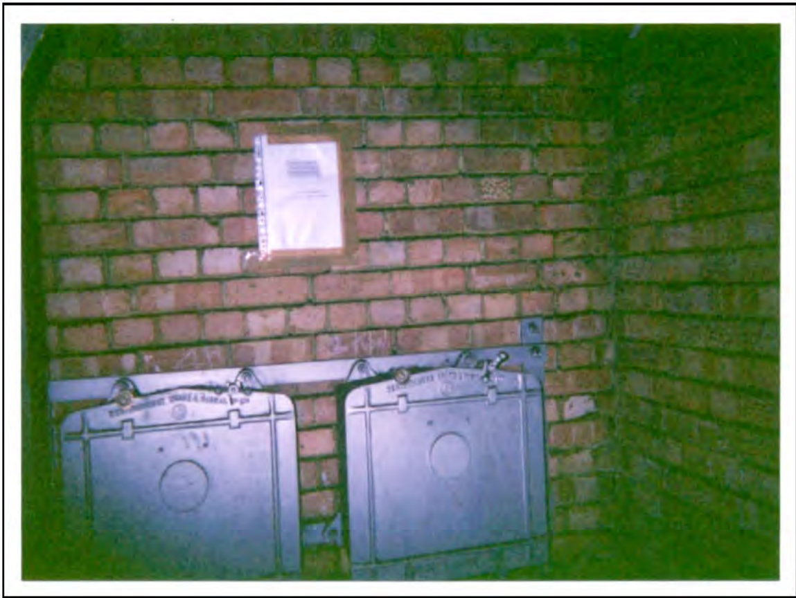
Figure 20: Material Strongly Presumed To Contain Asbestos
