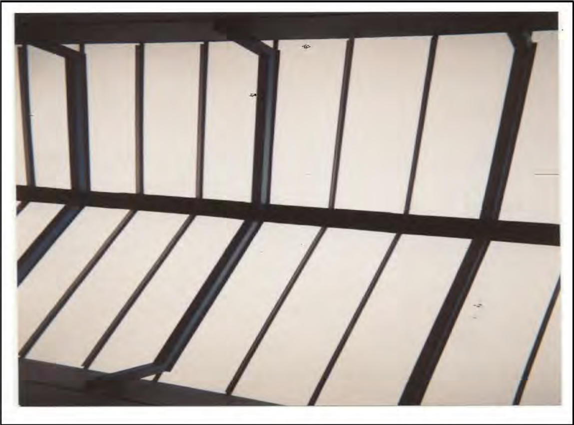
Figure 12: Material Strongly Presumed To Contain Asbestos
