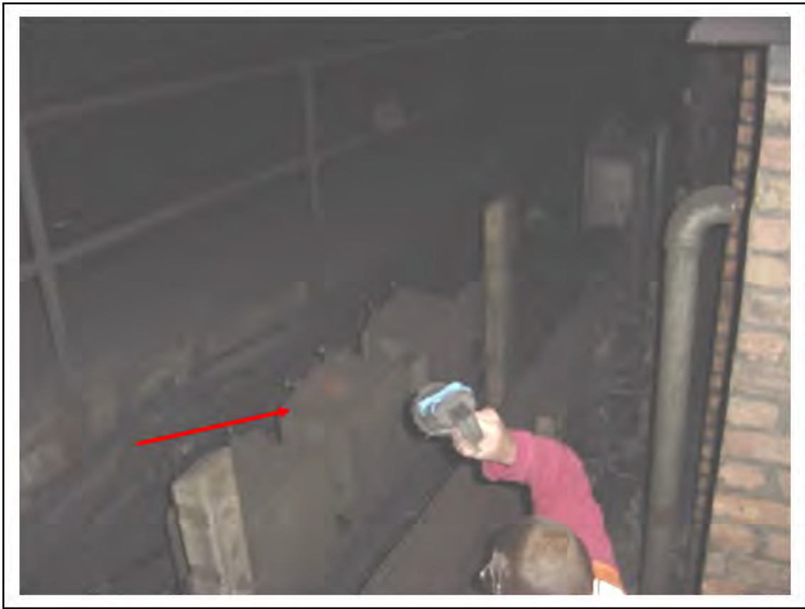
Figure 29: Material Strongly Presumed To Contain Asbestos
