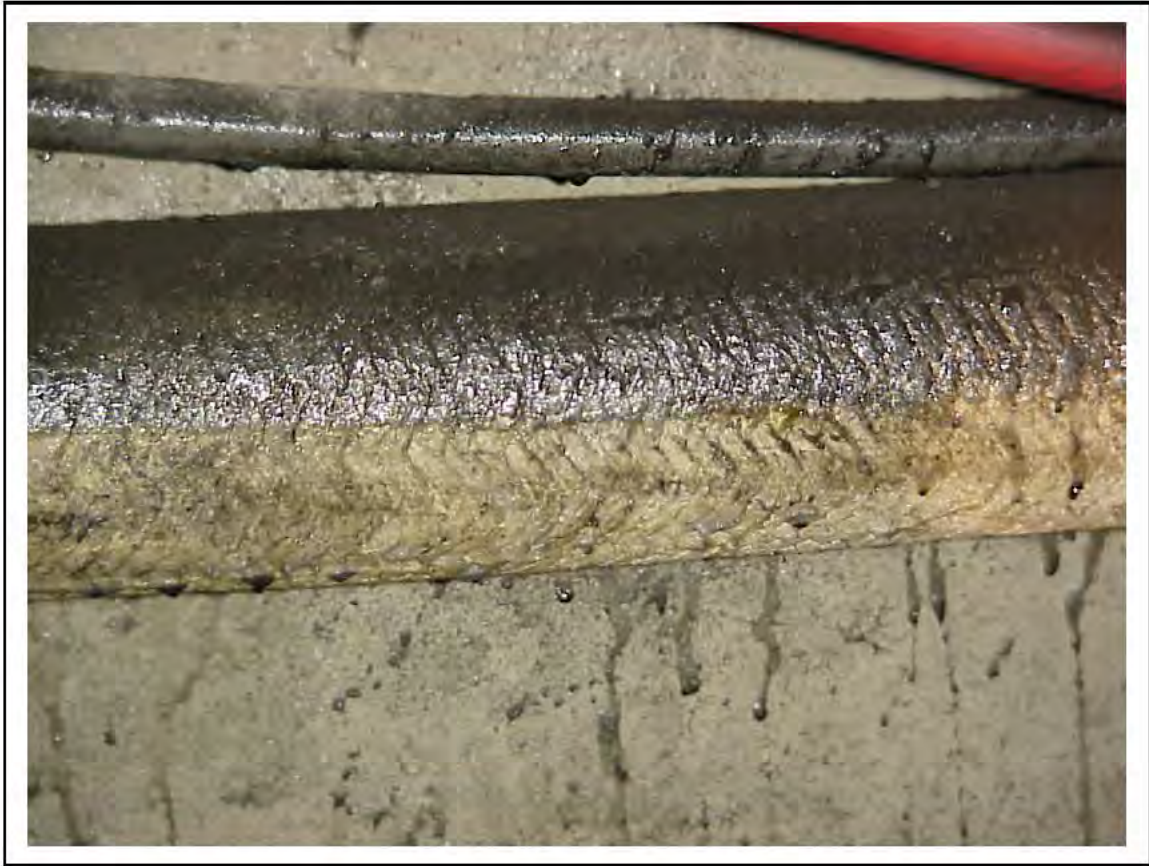
Figure 39: Material Strongly Presumed To Contain Asbestos
