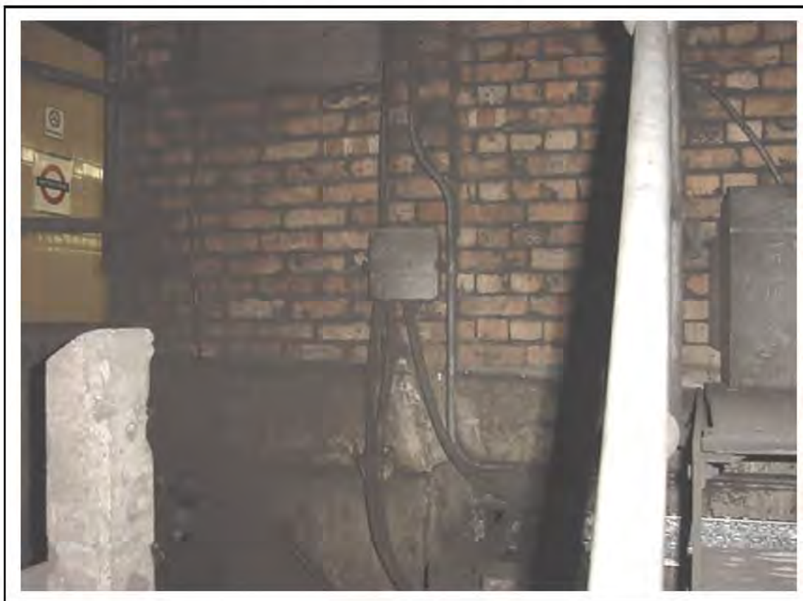
Figure 30: Material Strongly Presumed To Contain Asbestos
