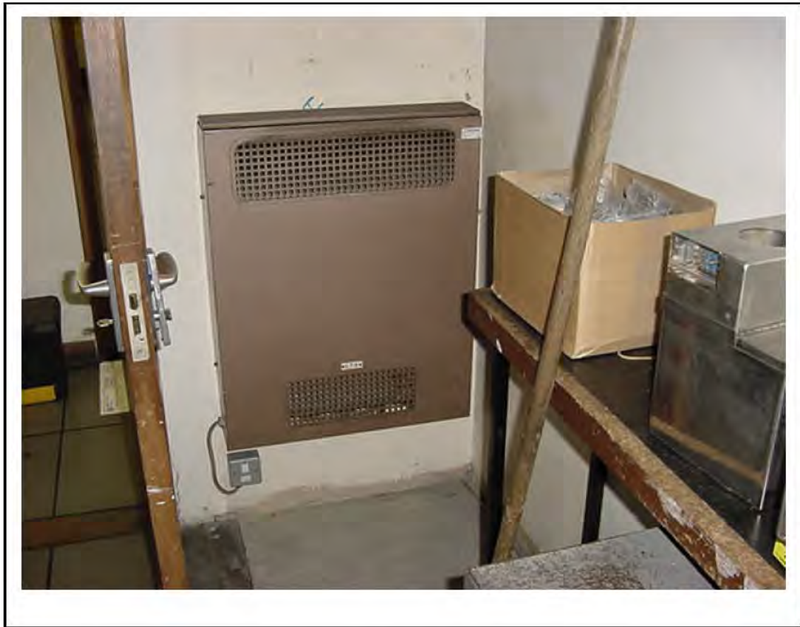
Figure 17: Material Strongly Presumed To Contain Asbestos
