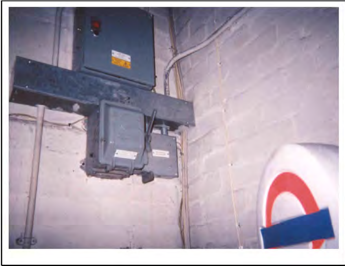
Figure 16: Material Strongly Presumed To Contain Asbestos
