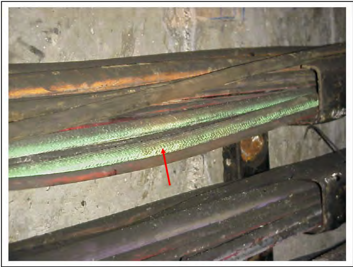
Figure 45: Material Strongly Presumed To Contain Asbestos
