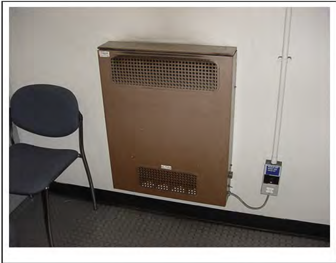
Figure 18: Material Strongly Presumed To Contain Asbestos
