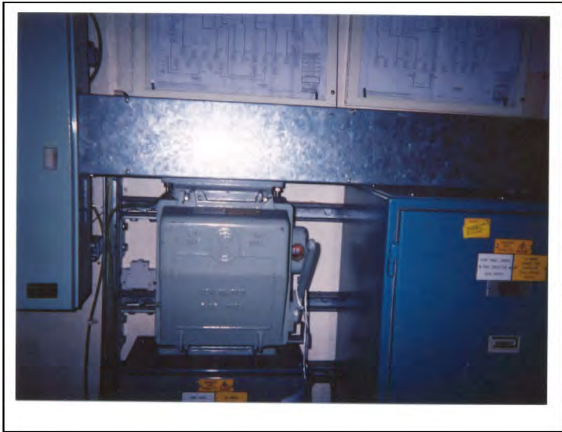
Figure 14: Material Strongly Presumed To Contain Asbestos
